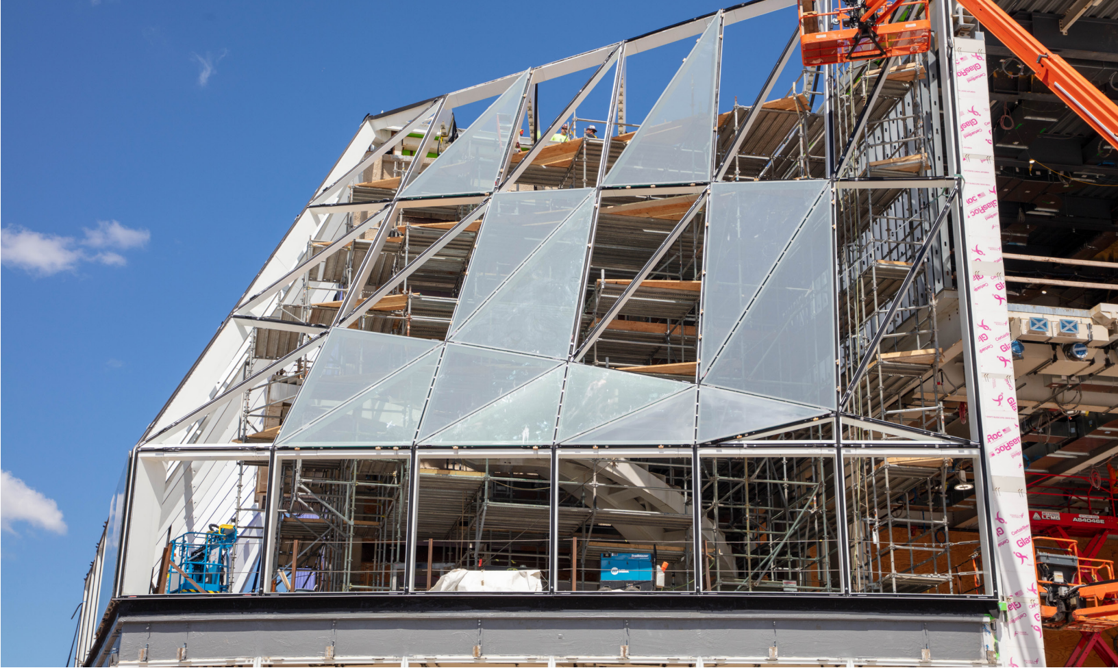
Installation of glass panels on the façade of the Jeffrey E. Gundlach Building. Photo: Jeff Mace
